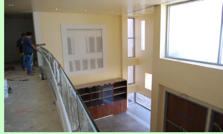
General Progress: Foyer balcony railing finishing up. Floor tile starts next week
