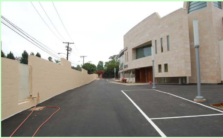
General Progress: Exterior asphalt road complete, lights installed, CMU wall painting underway
