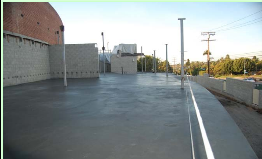
Exterior: 3rd floor concrete over metal deck poured! Steel to start Friday so as to get roof on.
