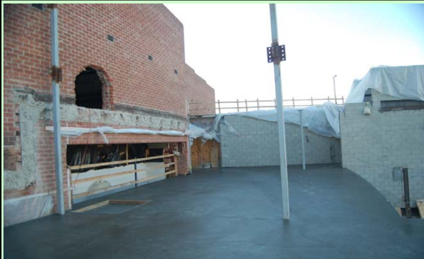
Exterior: 3rd floor concrete poured. To the left will be access to the library mezzanine
