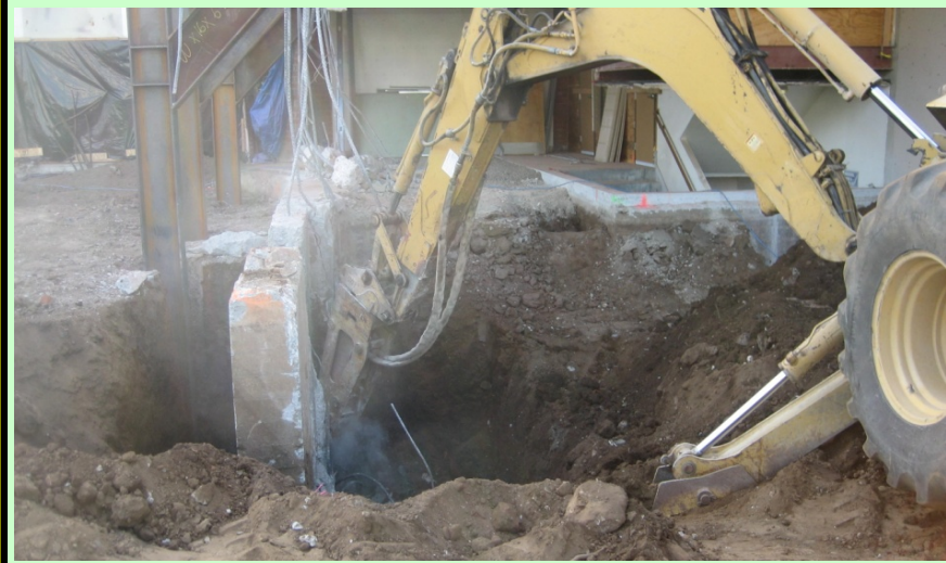
Exterior: Excavating for the new elevator pit and machine and electrical room.
