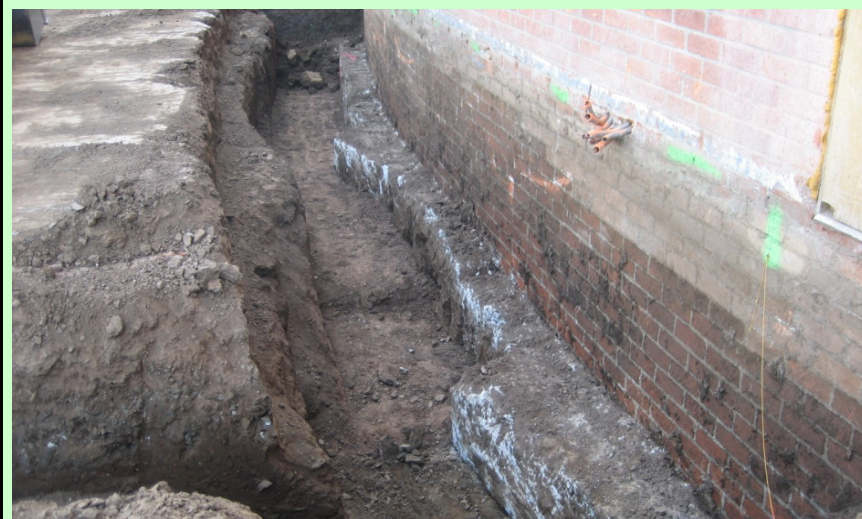
Exterior: Exposed existing footings along the sanctuary exterior wall. Construction in the 50's was a little different back then!
