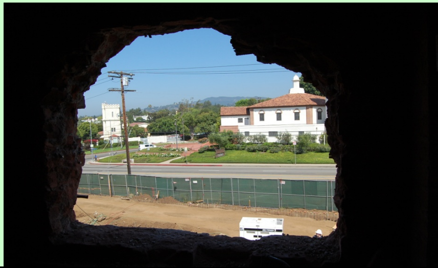
Exterior: Demolition to create tie-in of old structure with new for future library access.
