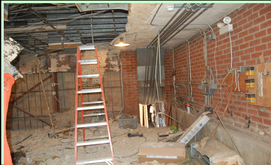
Interior: Demo of the "upper level" interior, where new library will be located.
