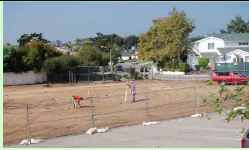
Exterior: Entryway site asphalt removed and surveying underway to lay out the new entry configuration
