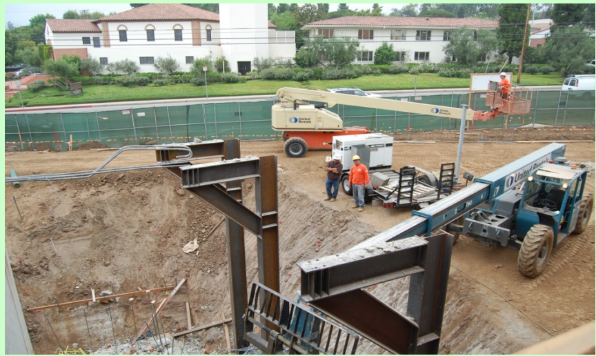
Exterior: Cleaning up the demo work. Notice the shoring is no longer holding up the 3rd floor now the CMU is built.
