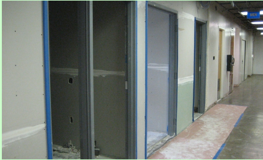
Interior: Bathroom / gift shop drywall taping - painting next week, followed by ceramic tile, then fixtures!. Doors to be hung.
