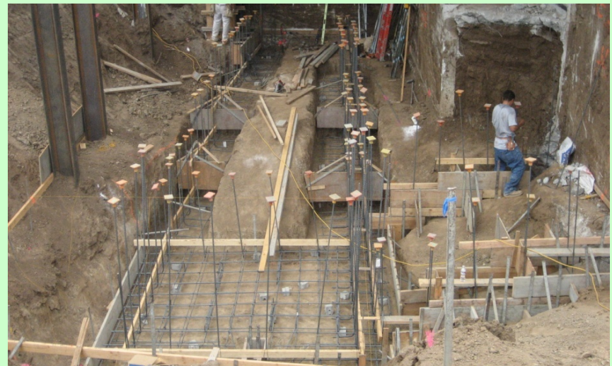
Exterior: Form and rebar for elevator pit and other walls in the basement level.
