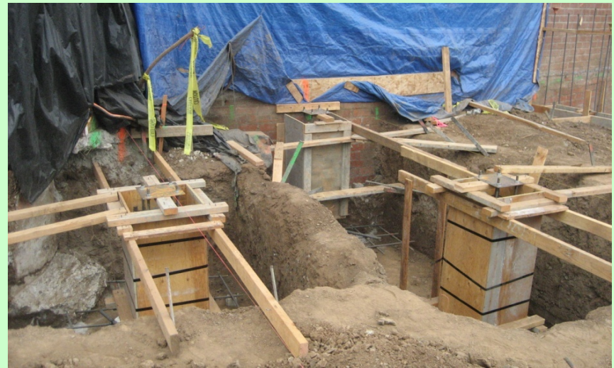
Exterior: Ongoing foundation work. Note steel column "brackets" are set on top. The steel columns will attach (bolts) to these.
